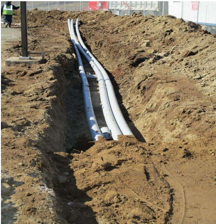
BURIED CONDUIT FOR EXISTING SCHOOL POWER
