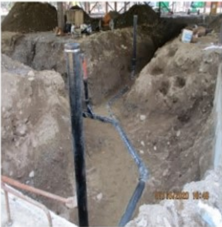
UNDERGROUND KITCHEN WASTE PIPING
